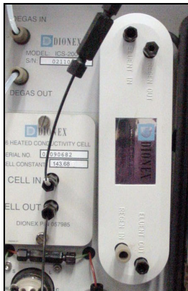
Figure B-20. Suppressor Installed (SRS Shown)
